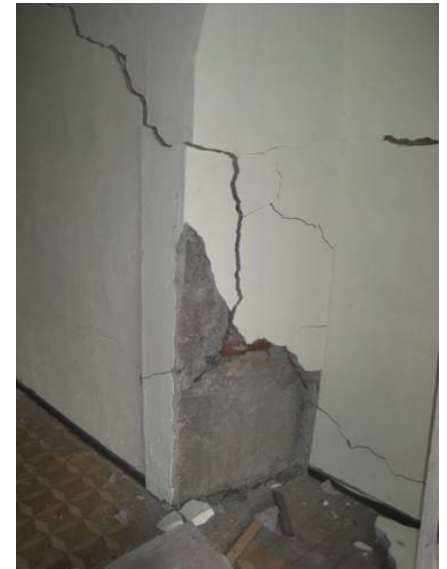
Some of the structural damage seen in the Bible Institute walls.
